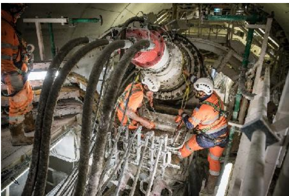
Planetary gearboxes as a screw conveyor drive on a tunnel boring machine
